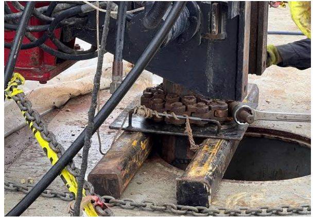
Photo 8 View of lift boat moonpool where sediment samples obtained utilizing sonic drill rig.
